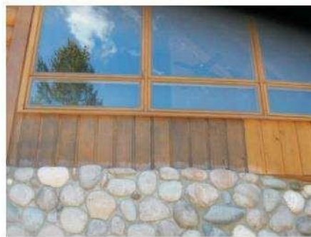
Section on left was wire brushed.
